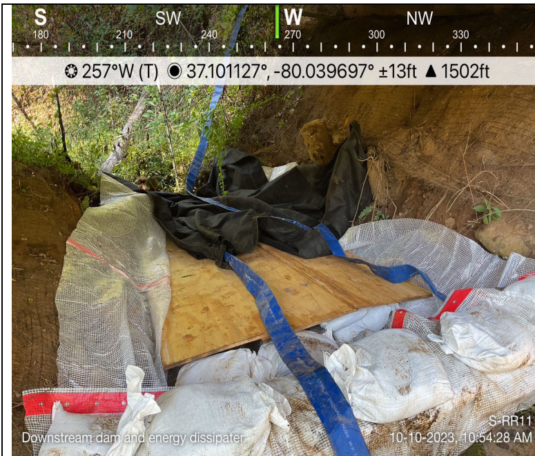
Photo Description: Energy dissipater.
