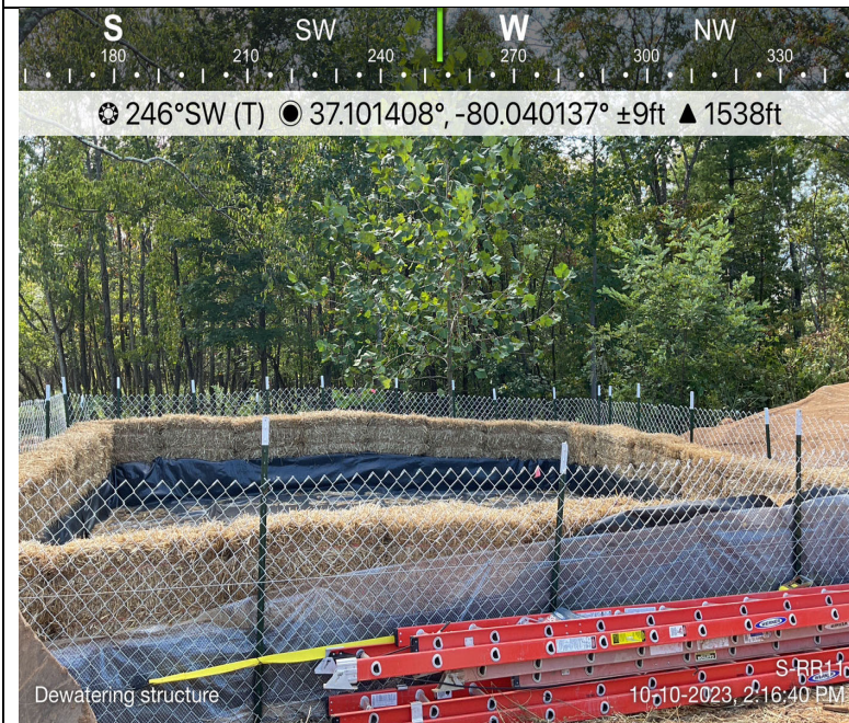
Photo Description: Dewatering structure.
