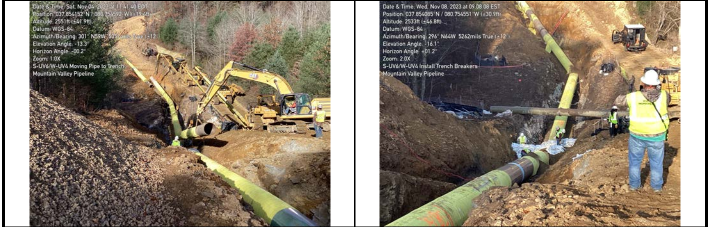
GPS Location See Photo GPS Location See Photo Description Photo 5: Lowering pipe into trench. Description Photo 6: Building trench breakers adjacent to aquatic resource area.
