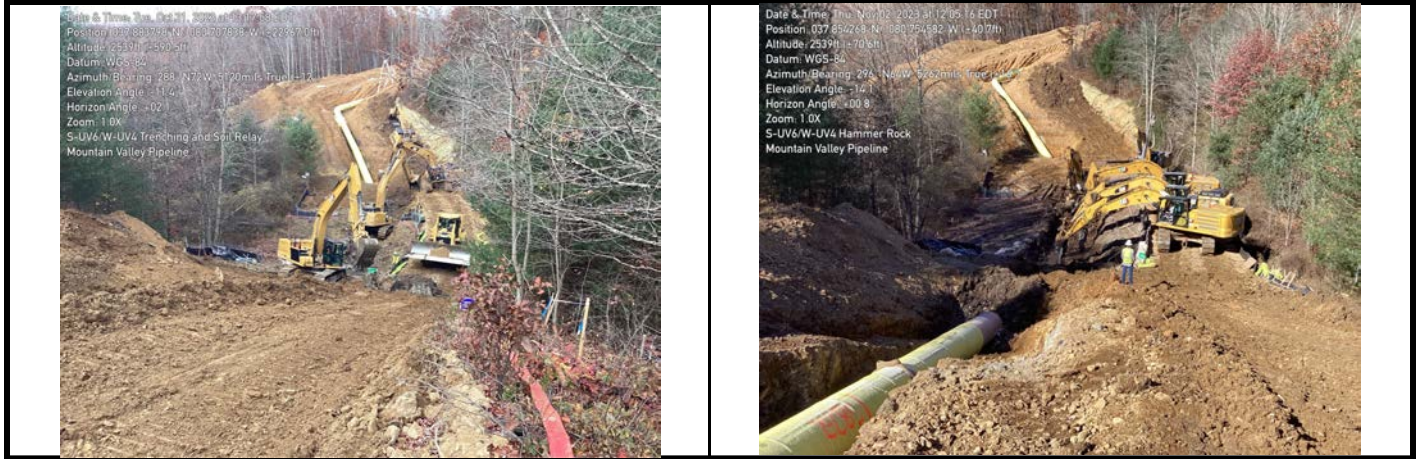
GPS Location See Photo GPS Location See Photo Description Photo 3: Trenching through aquatic resource. Description Photo 4: Hammering rock in aquatic resource area.
