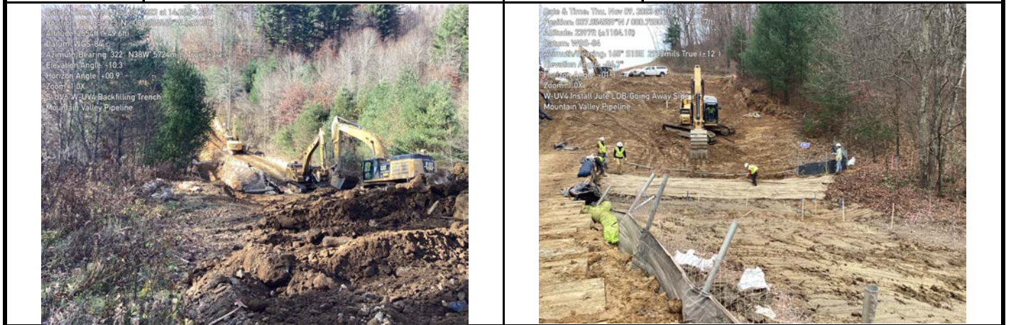
GPS Location See Photo GPS Location See Photo Description Photo 7: Backfilling of resource area. Description Photo 8: Jute installed on LDB of stream.
