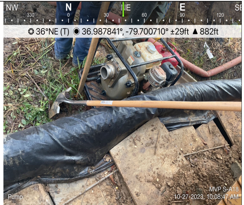
Photo Description: Dam and pumps installed on-site for stream and wetland crossing.
