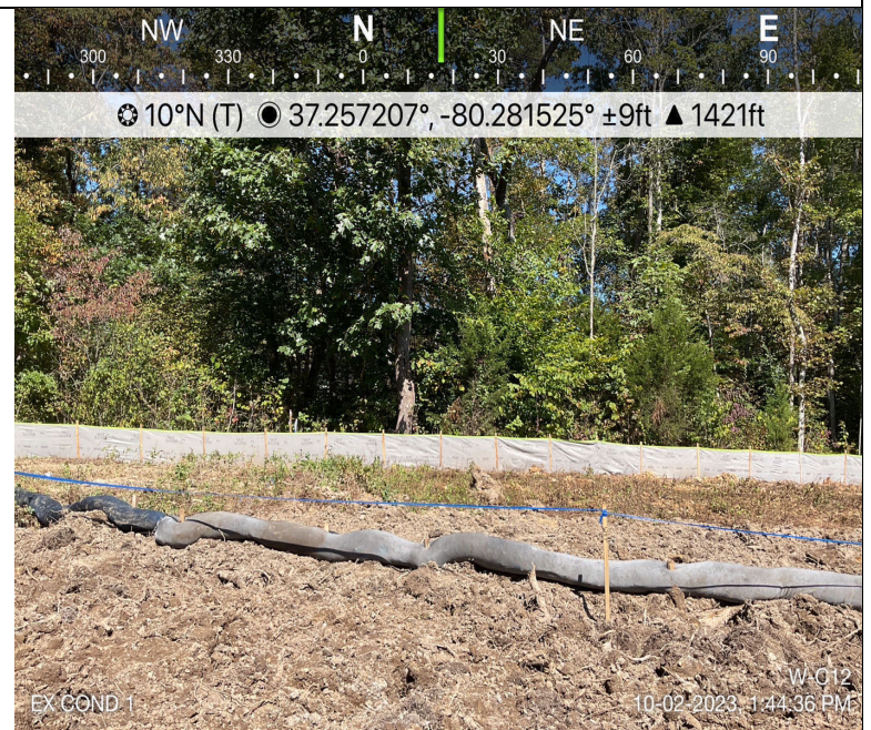
Photo Description: At edge of LOD, view of unpermitted resource area conditions during post-construction assessment.
