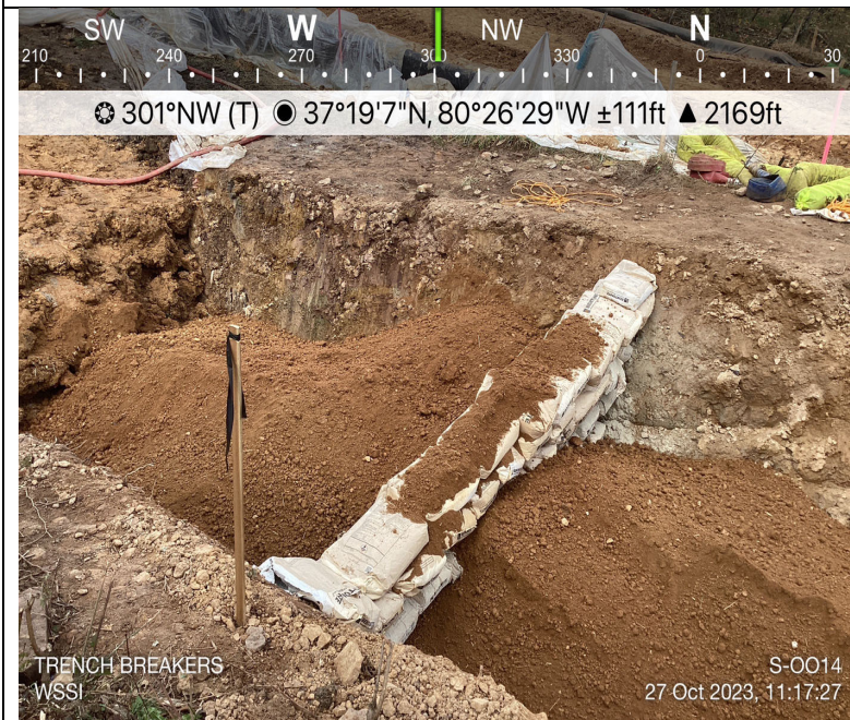
Photo Description: Trench breakers installed at stream/wetland crossing. Stream S-0014 is directly adjacent to wetland W-CD12.
