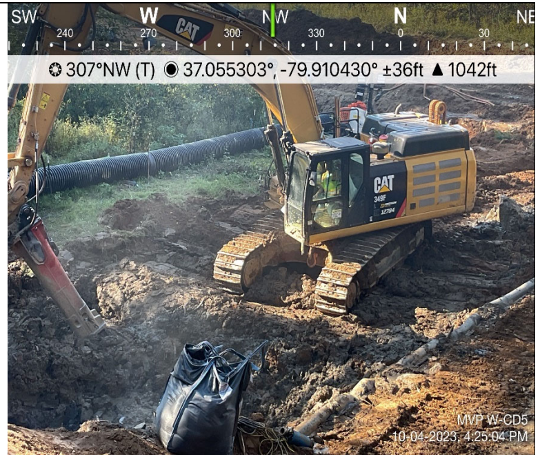
Photo Description: Excavator within wetland area on timber mats. No geotextile fabric observed under timber mats. DEQ reported. No unauthorized discharge or impacts to biological conditions observed.
