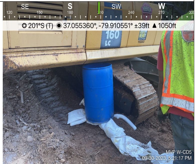
Photo Description: Petroleum spill clean up and disposal of contaminated material. No unauthorized discharge or impacts to biological conditions observed.
