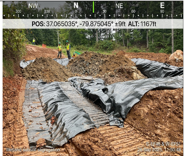
Photo Description: Wetland topsoil stockpiled and staged separately from sub soil and other soils.
