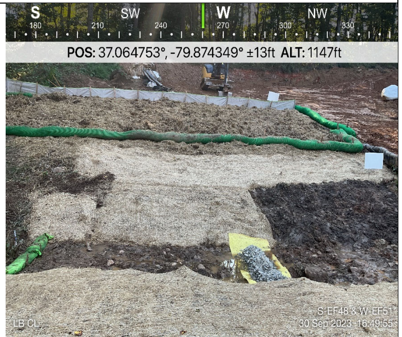
Photo Description: Restoration mostly completed, and check dams remain installed to assist with settling turbidity from restoring streamflow to impact area.
