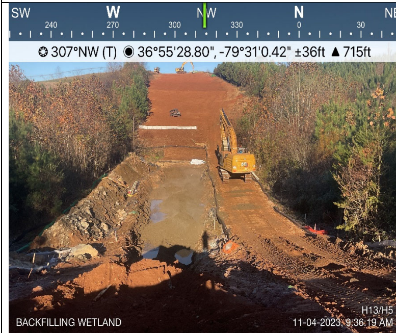
Photo Description: An overview of the wetland as it is being backfilled.
