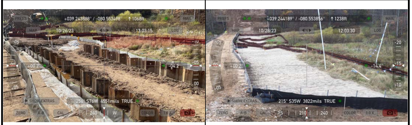
GPS Location See photo GPS Location See photo Description This photo shows the backfilled trench through the stream/wetland complex Description This photo shows the restored wetland
