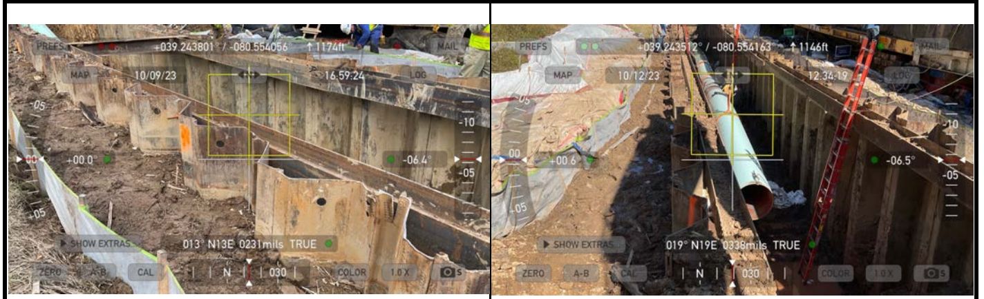
GPS Location See photo GPS Location See photo Description This photo shows the excavated trench through the stream/wetland complex Description This photo shows the contractor working on installing the pipe
