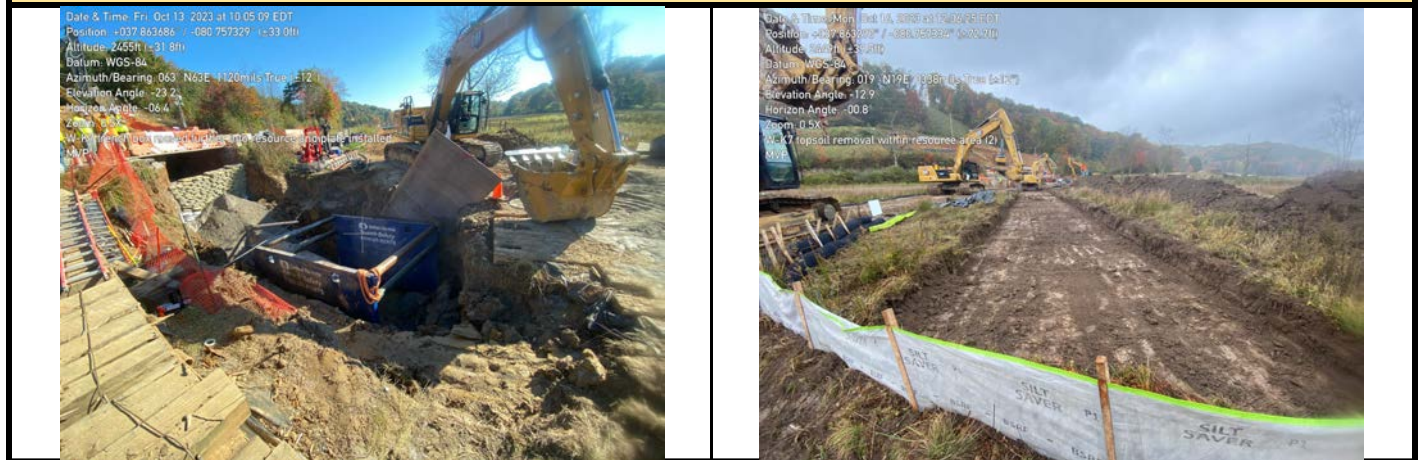
GPS Location See Photo GPS Location See Photo Description Photo 3: Concrete trench breakers under construction, filling trench, and moving trench box and plates. Description Photo 4: Removal of topsoil from remaining wetland area.
