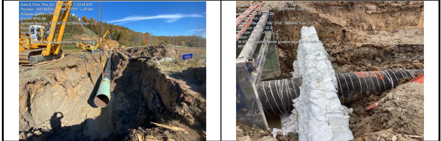
GPS Location See Photo GPS Location See Photo Description Photo 5: Placing and positioning pipe through aquatic resource area. Description Photo 6: Downgradient (southern) trench breaker adjacent to aquatic resource.
