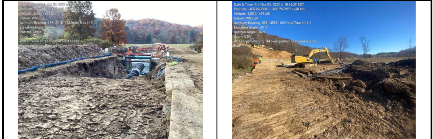
GPS Location See Photo GPS Location See Photo Description Photo 7: Backfilling of aquatic resource. Description Photo 8: Replacing timber mats and restoring wetland topsoil.
