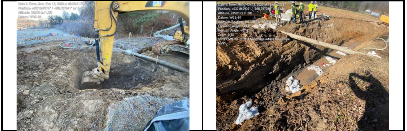
GPS Location See Photo GPS Location See Photo Description Photo 3: Excavating trench in aquatic resource area. Equipment on timber mats. Description Photo 4: Adding sandbag padding to trench in aquatic resource area.
