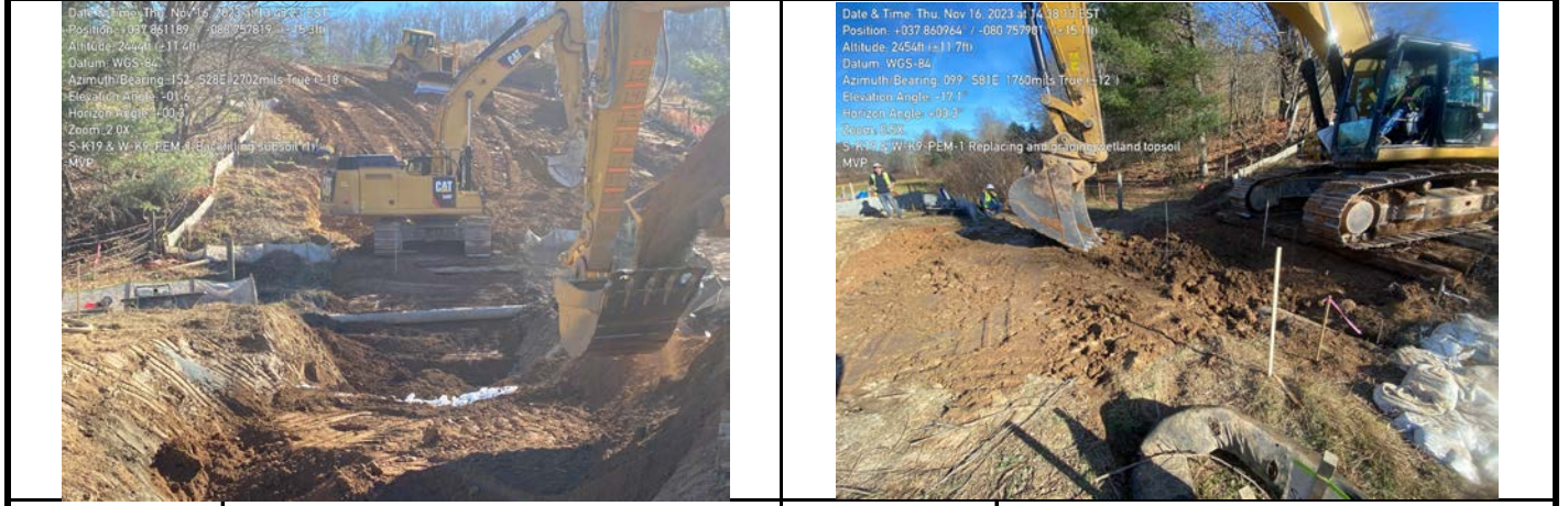
GPS Location See Photo GPS Location See Photo Description Photo 7: Backfilling in aquatic resource area. Description Photo 8: Restoring and grading wetland topsoil.
