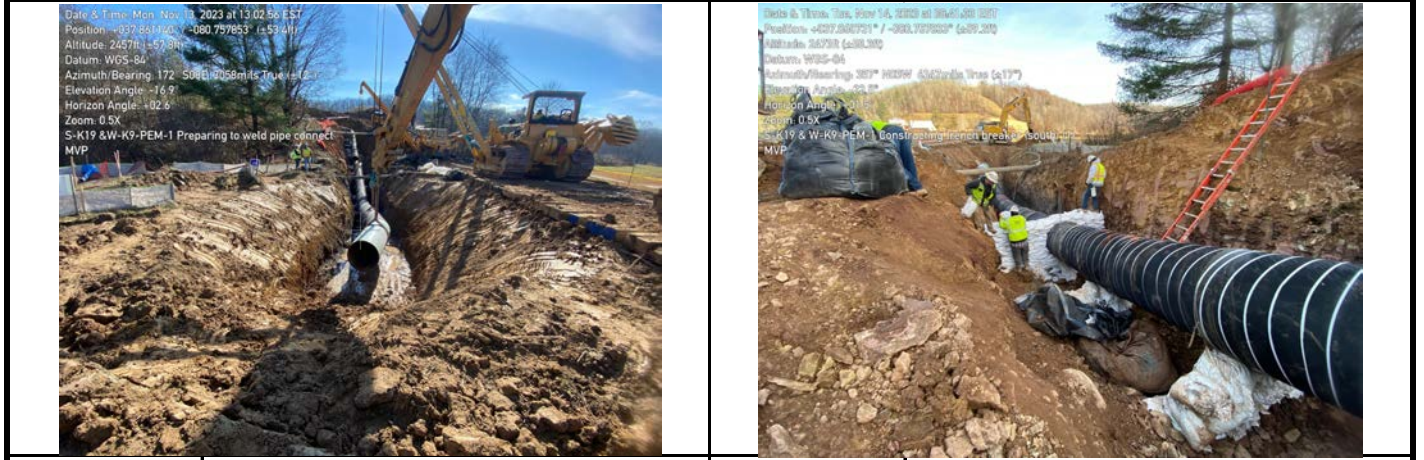
GPS Location See Photo GPS Location See Photo Description Photo 5: Lowering pipe into trench through aquatic resource area and preparing for welding. Description Photo 6: Construction of trench breaker on the southern side of aquatic resource area.
