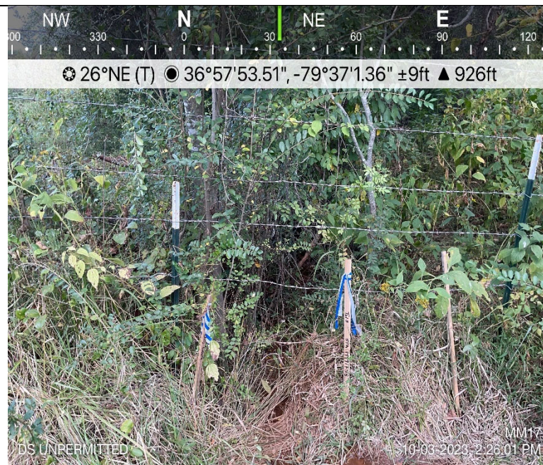
Photo Description: At edge of LOD, view of unpermitted resource area conditions during post-construction assessment. Delineation indicates W-MM17 converges with S-D7 within temporary impact area.
