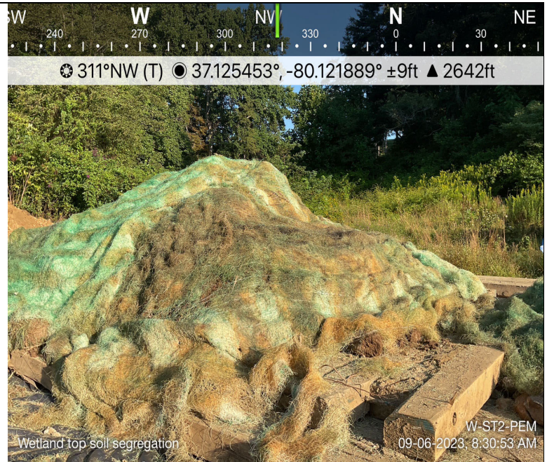
Photo Description: Wetland topsoil segregated and stockpiled separately from subsoil and S-G24 & S-G25 streambed substrate.
