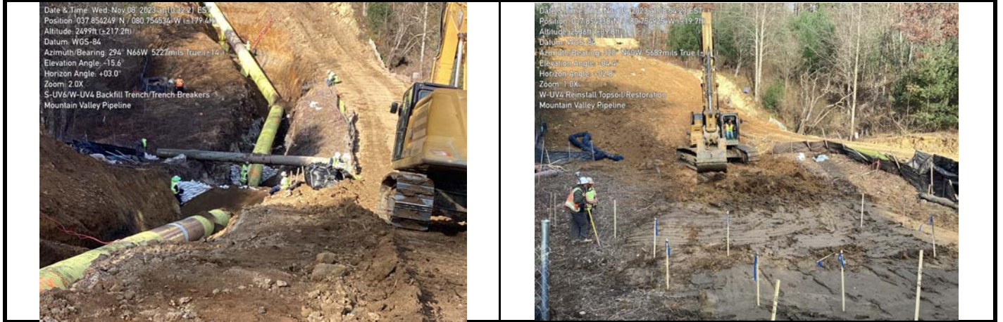
GPS Location See Photo GPS Location See Photo Description Photo 7: Trench breakers and backfilling with padding dirt. Description Photo 8: Restoring wetland topsoil.
