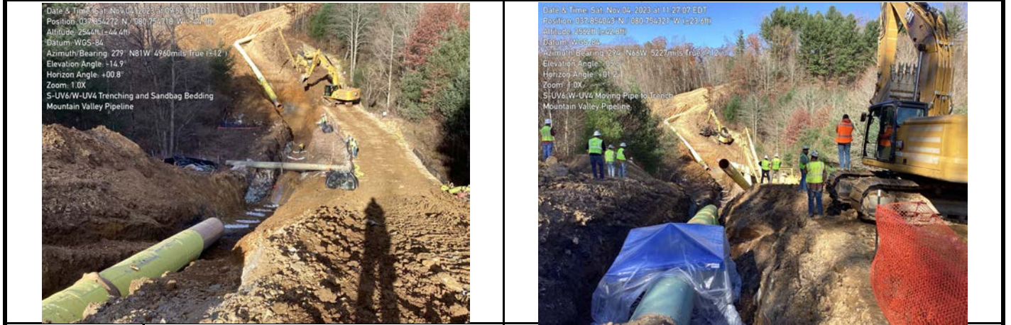
GPS Location See Photo GPS Location See Photo Description Photo 5: Sandbags in trench for pipe bedding. Description Photo 6: Lowering pipe into trench.
