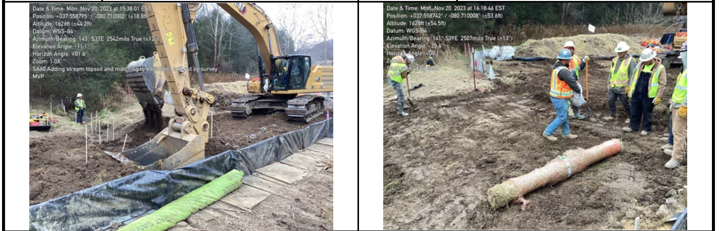
GPS Location See Photo GPS Location See Photo Description Photo 7: Adding topsoil and contouring to meet elevations. Description Photo 8: Spreading seed in buffer.
