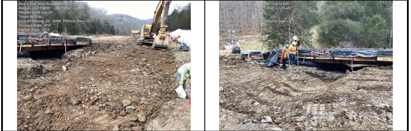
GPS Location See Photo GPS Location See Photo Description Photo 5: Shaping subsoil. Description Photo 6: Survey shooting elevations.
