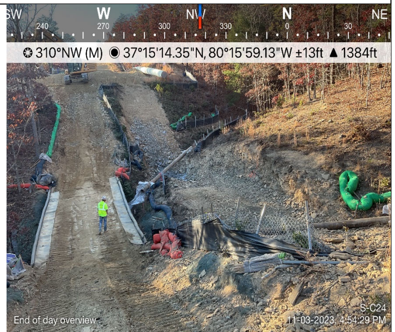
Photo Description: Conditions of the resource impact area at the end of a workday. Flume remains installed and operational.
