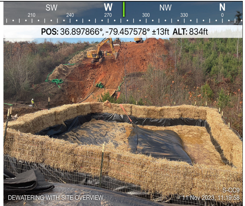
Photo Description: An overview of the dewatering structure installed on the GAS.
