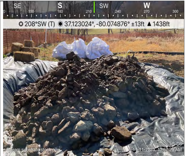
Photo Description: Stream substrate and stream cobble stockpiled on timber mats and geotech outside of the 50-foot buffer.
