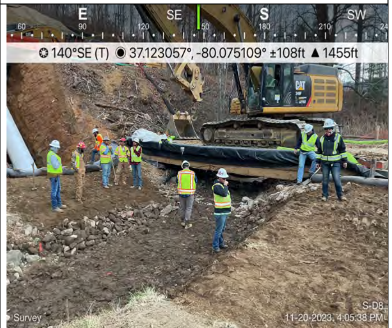
Photo Description: Survey shooting the final grade for the stream and banks within the 10-foot buffer.
