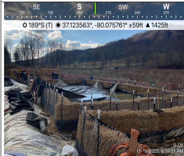
Photo Description: Dewatering structures used for filtering ground water from the trench.
