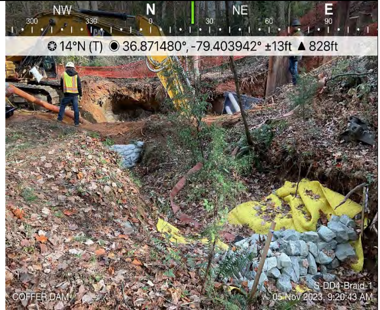
Photo Description: The dam and pump energy dissipation device was installed and maintained throughout the crossing.
