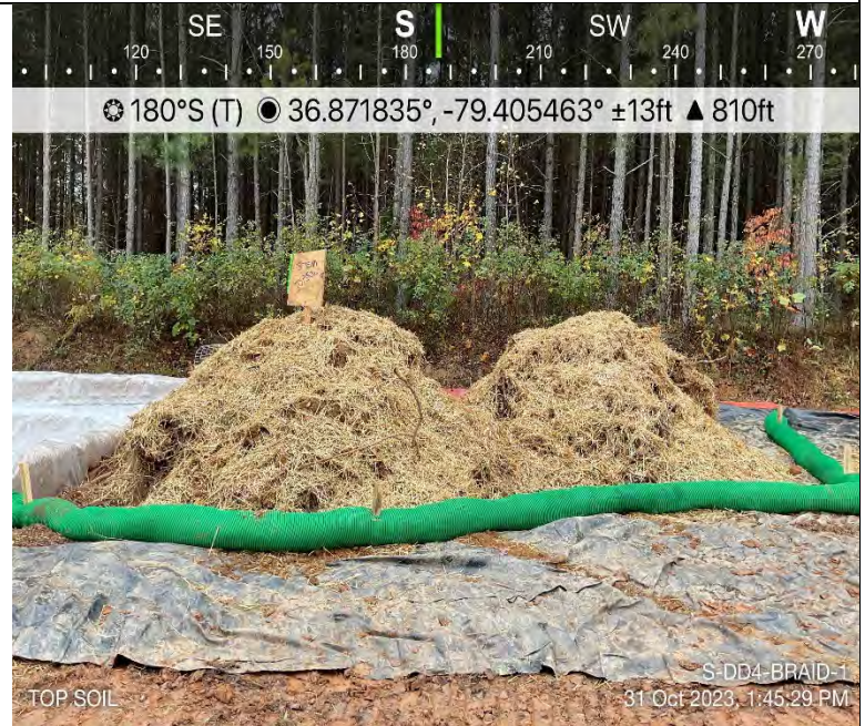
Photo Description: The streambed material was stockpiled separately from subsoil in the upland area on a geotextile liner.
