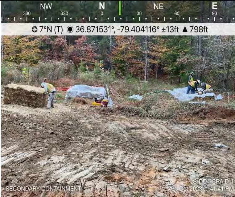
Photo Description: The crew installing secondary containment to be used during construction.
