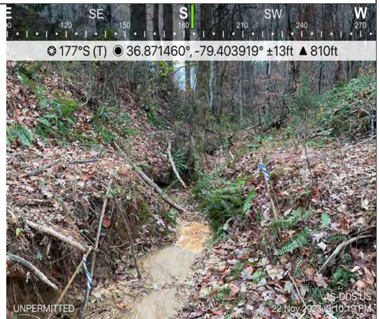
Photo Description: Conditions of the downstream area outside the ROW during post-construction assessment. Site appears different due to landowner modifications and construction activities since 2018.
