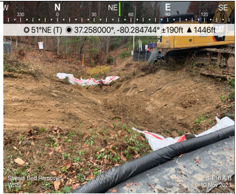
Photo Description: Streambed and buffer zone topsoil removed and stockpiled separately prior to subsoil excavation.
