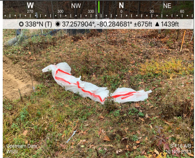
Photo Description: Upstream dam installed and operating prior to in-stream work activity.
