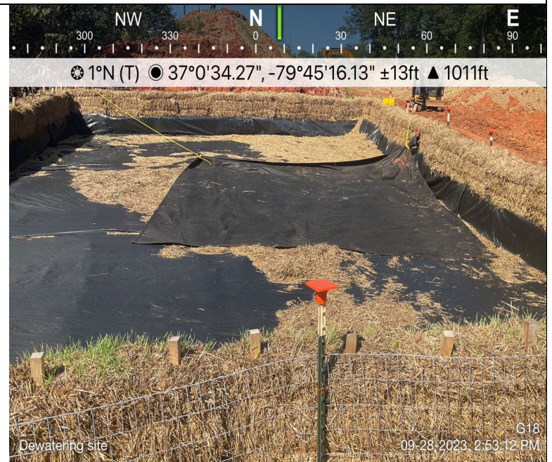
Photo Description: Dewatering area
