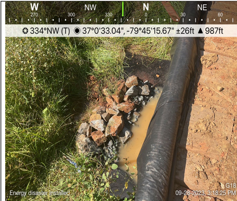
Photo Description: Energy dissipater
