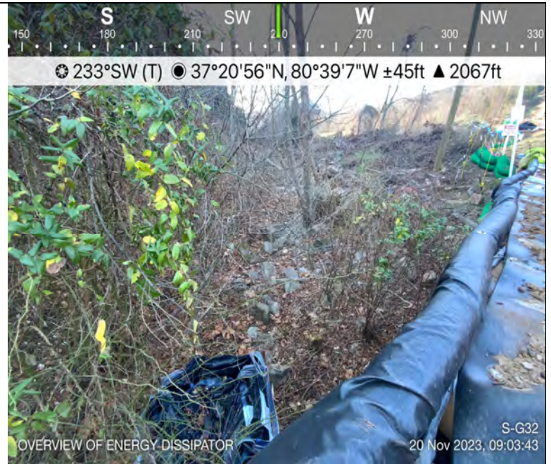
Photo Description: An overall view of the energy dissipator, dam, and pump set up under the timber mat bridge.
