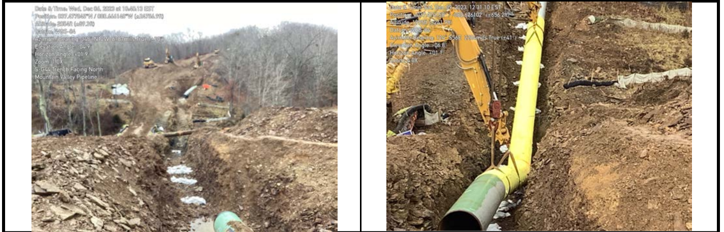
GPS Location See Photo GPS Location See Photo Description Photo 3: Trench completed in aquatic resource. Description Photo 4: Lowering pipe into trench.
