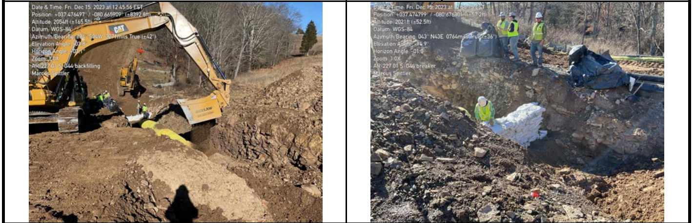
GPS Location See Photo GPS Location See Photo Description Photo 5: Backfilling. Description Photo 6: Constructing trench breaker.
