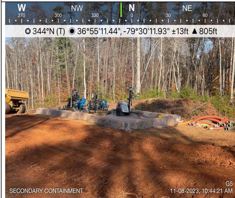
Photo Description: Secondary containment for light plants and pumps.
