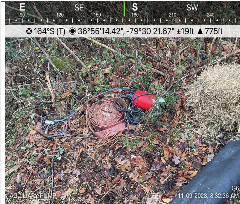
Photo Description: Auxiliary pump
