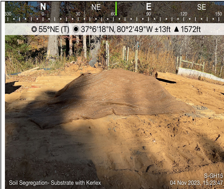
Photo Description: Soil Segregation - Substrate under erosion control matting.
