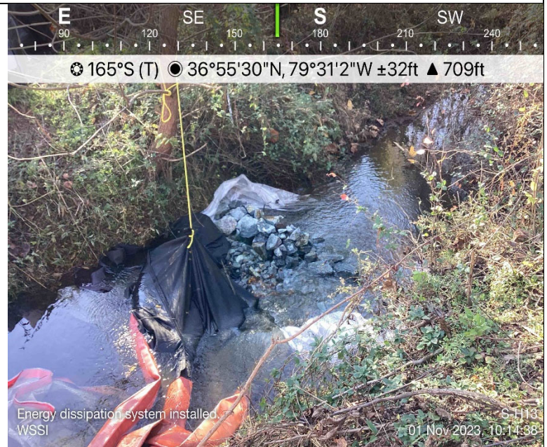
Photo Description: Energy dissipation for pump around
