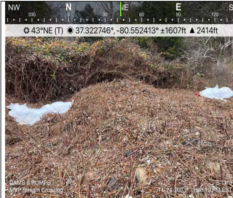
Photo Description: Dam and pump installed and available for operation throughout crossing.
