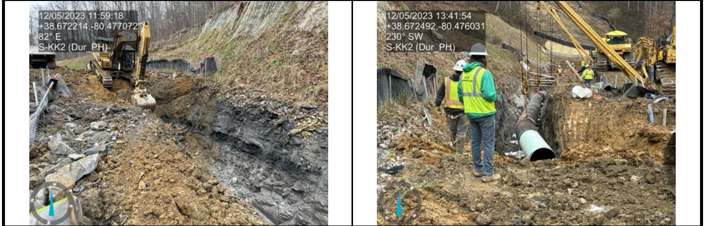
GPS Location See Photo GPS Location See Photo Description Excavation of the rock layer through S-KK2. Description Lowered in a section of pipe through S-KK2.
