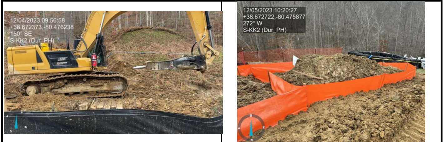
GPS Location See Photo GPS Location See Photo Description Using timber mats while rock hammering through S-KK2. Description Segregation of the top 12" of stream bank soil.
