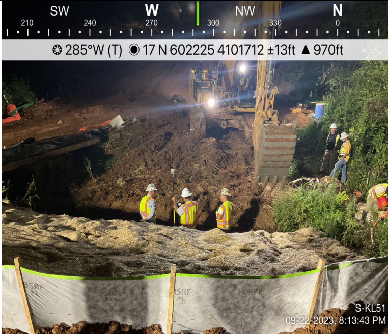
Photo Description: The survey crew providing levels to assist in the stream restoration.
