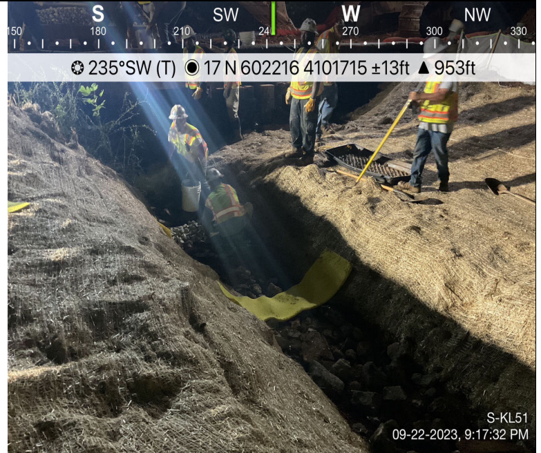
Photo Description: The crew in the process of removing the rock check dam after restoration was complete.
