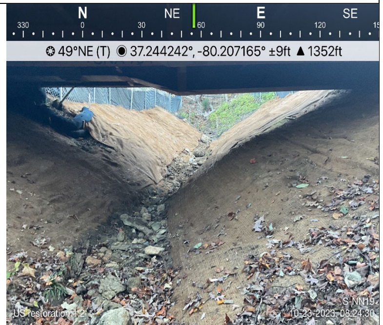
Photo Description: Conditions of the downstream area outside the impact area under the bridge during post-construction assessment.
