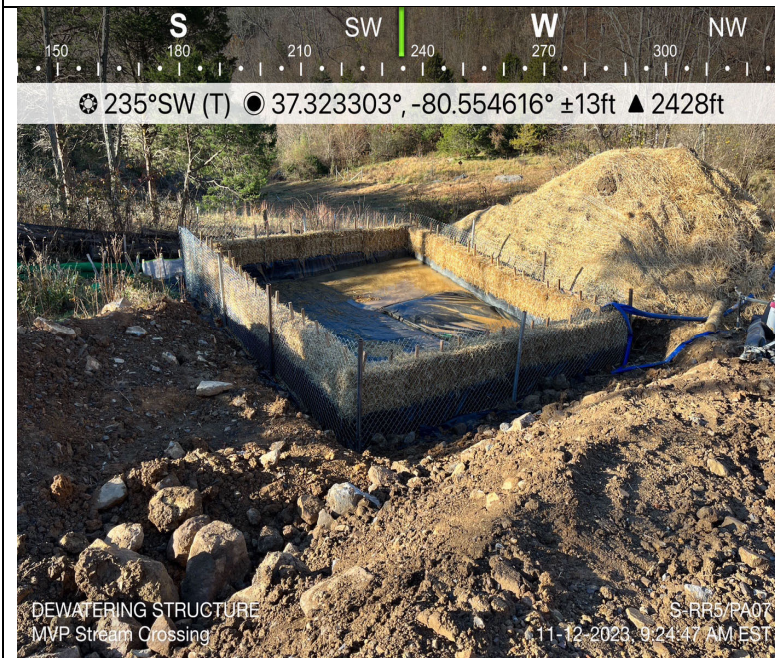
Photo Description: De-watering structure
