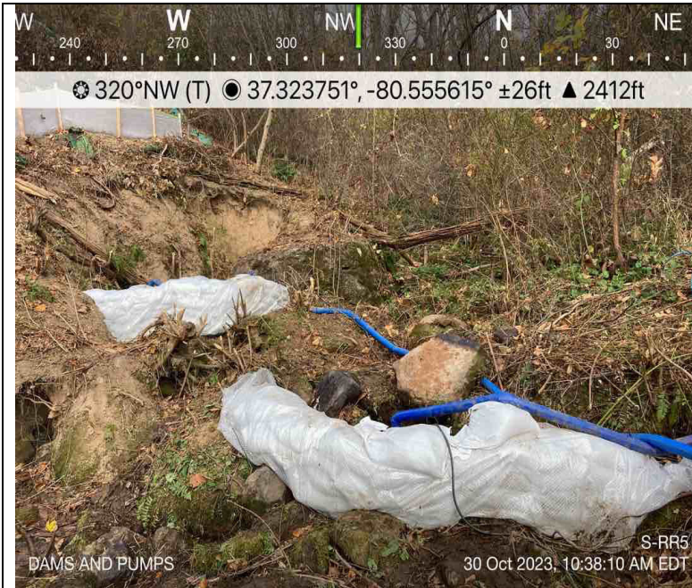
Photo Description: Dams & pumps
