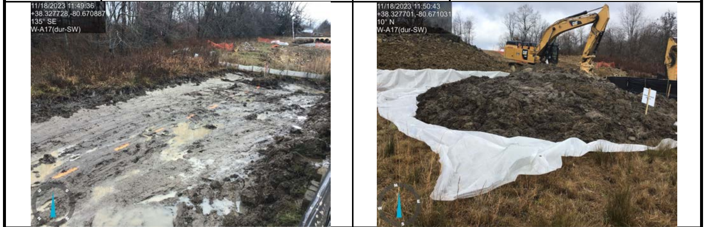
GPS Location See coordinates in above photo. GPS Location See coordinates in above photo. Description Topsoil being removed from wetland area. Description Wetland topsoil staged on plastic and segregated from other spoils on the CIS of resource.
