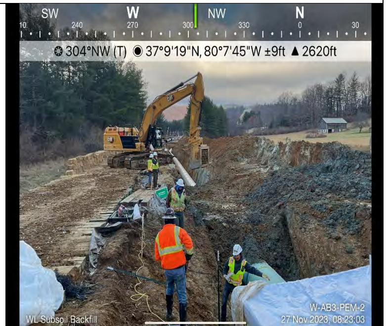
Photo Description: Backfill of subsoil through wetland impact area after pipe installation.
