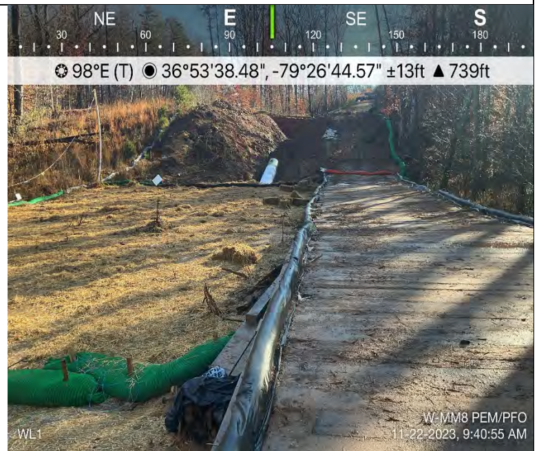
Photo Description: Conditions of wetland area post-restoration. Timber mat bridges remain installed across resources for access to upland areas for project completion.
