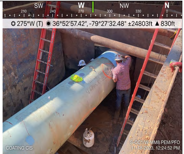
Photo Description: Coating completed for weld on coming in side of the resources after QA/QC of welds.
