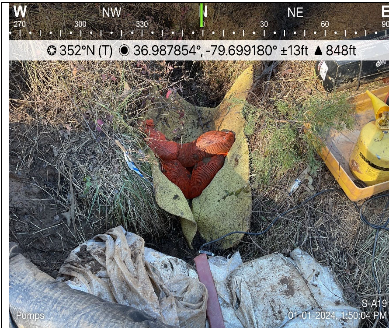
Photo Description: The dam was installed and the pump around was functioning as designed.
