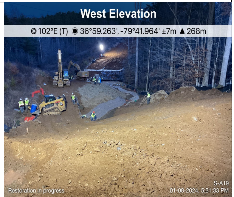
Photo Description: An overview of the site restoration. Crews installing new ESCs, applying riparian seed, stabilization matting, and straw.
