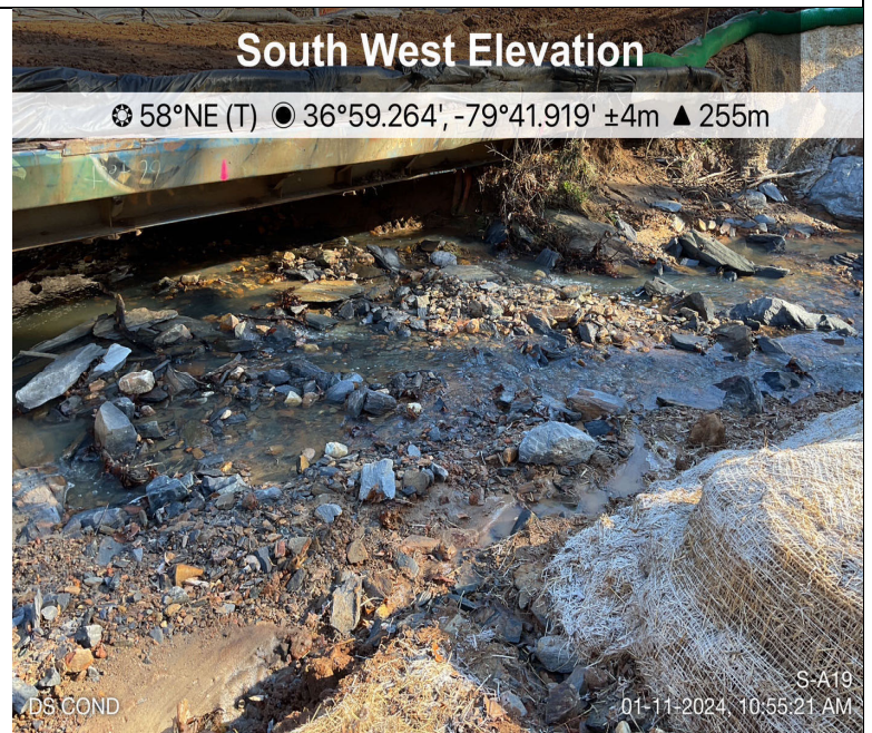
Photo Description: Conditions of the downstream area outside the ROW during post-construction assessment. S-A19-H26 converges with S-A20 within the permitted impact area.
