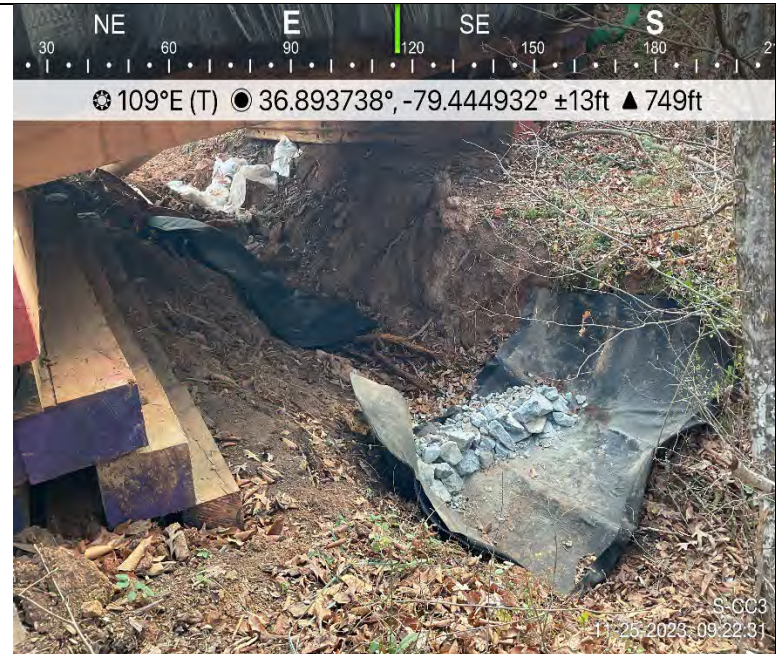
Photo Description: A flume and energy dissipator installed within the resource.
