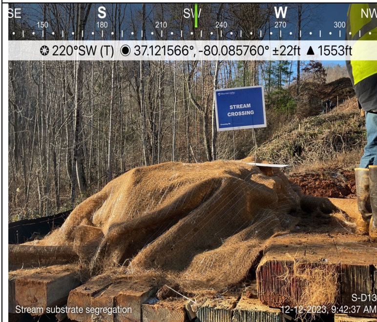
Photo Description: The top 12-inches of stream substrate was segregated and stabilized.
