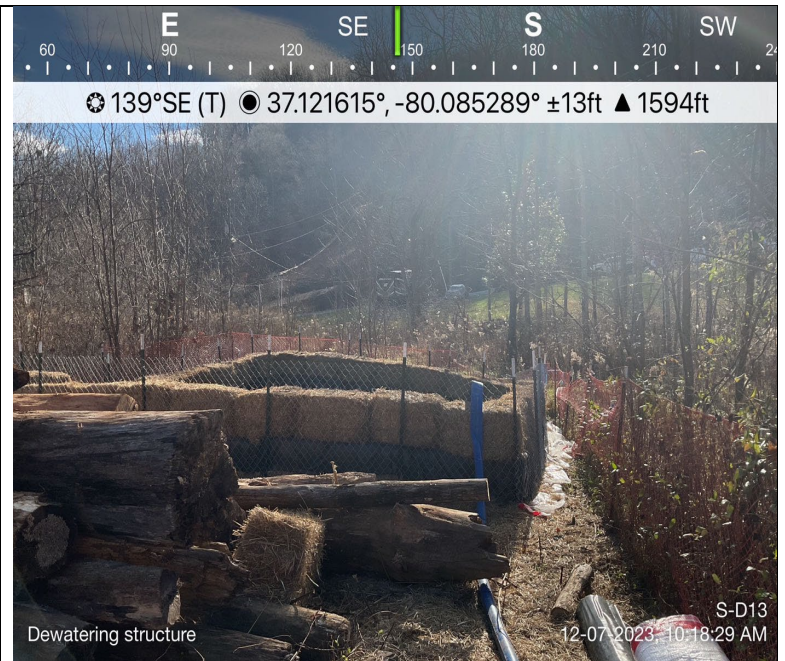
Photo Description: An overview of the dewatering structure functioning as designed.
