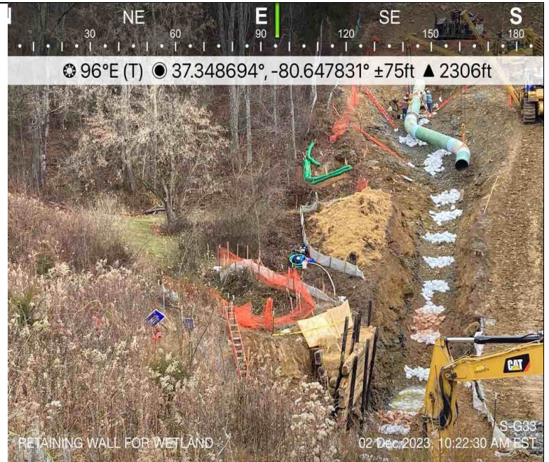
Photo Description: A retaining wall was constructed to prevent sloughing of the adjacent manmade pond into the resource.
