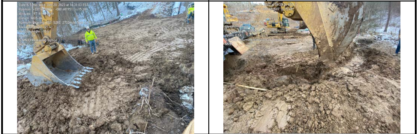
GPS Location See Photo GPS Location See Photo Description Photo 7: Restoring topsoil. Description Photo 8: Restoring substrate.
