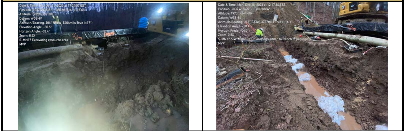
GPS Location See Photo GPS Location See Photo Description Photo 3: Excavating through aquatic resource. Description Photo 4: Placing sandbags in trench for padding.
