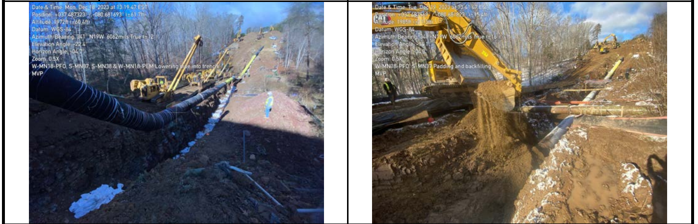
GPS Location See Photo GPS Location See Photo Description Photo 5: Putting pipe in trench through aquatic resource area. Description Photo 6: Adding padding and backfilling.
