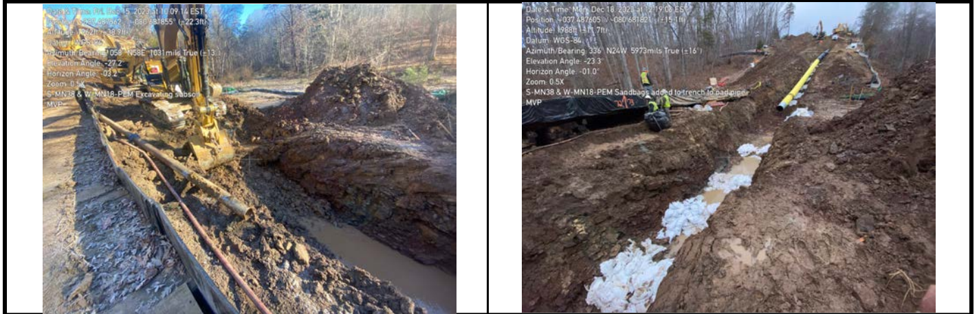
GPS Location See Photo GPS Location See Photo Description Photo 3: Excavation of trench through aquatic resource. Description Photo 4: Sandbags in trench for padding.
