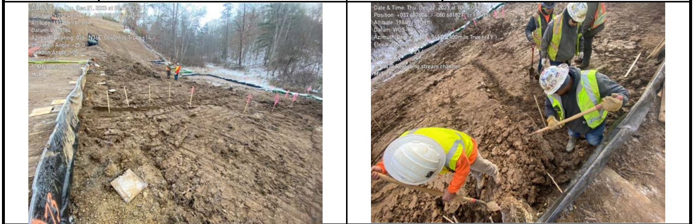
GPS Location See Photo GPS Location See Photo Description Photo 7: Elevations staked by survey. Description Photo 8: Contouring channel by hand.
