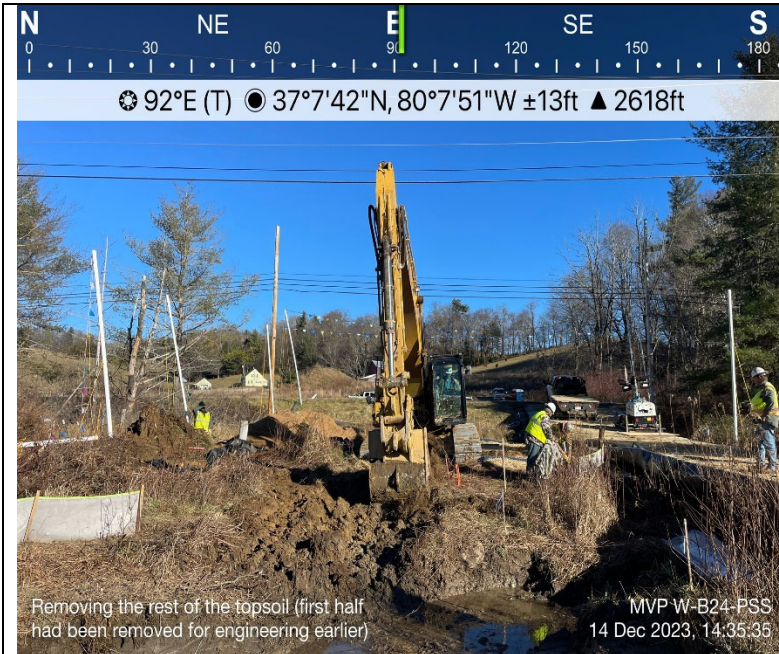
Photo Description: Removal of top 12 inches of wetland topsoil for separate storage and stabilization.
