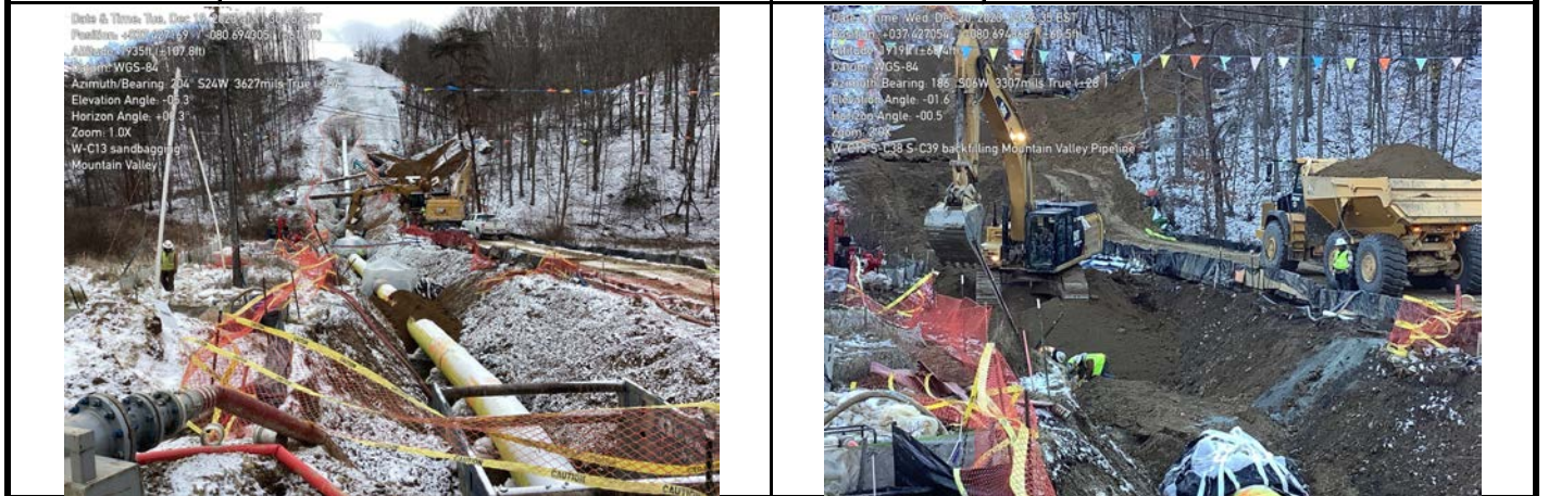
GPS Location See Photo GPS Location See Photo Description Photo 5: Padding and sandbags in trench. Description Photo 6: Backfilling of trench.
