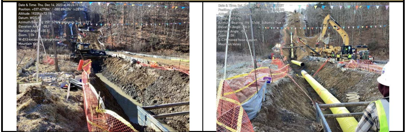
GPS Location See Photo GPS Location See Photo Description Photo 3: Excavating through aquatic resource. Description Photo 4: Pipe lowered into trench into aquatic resource area.
