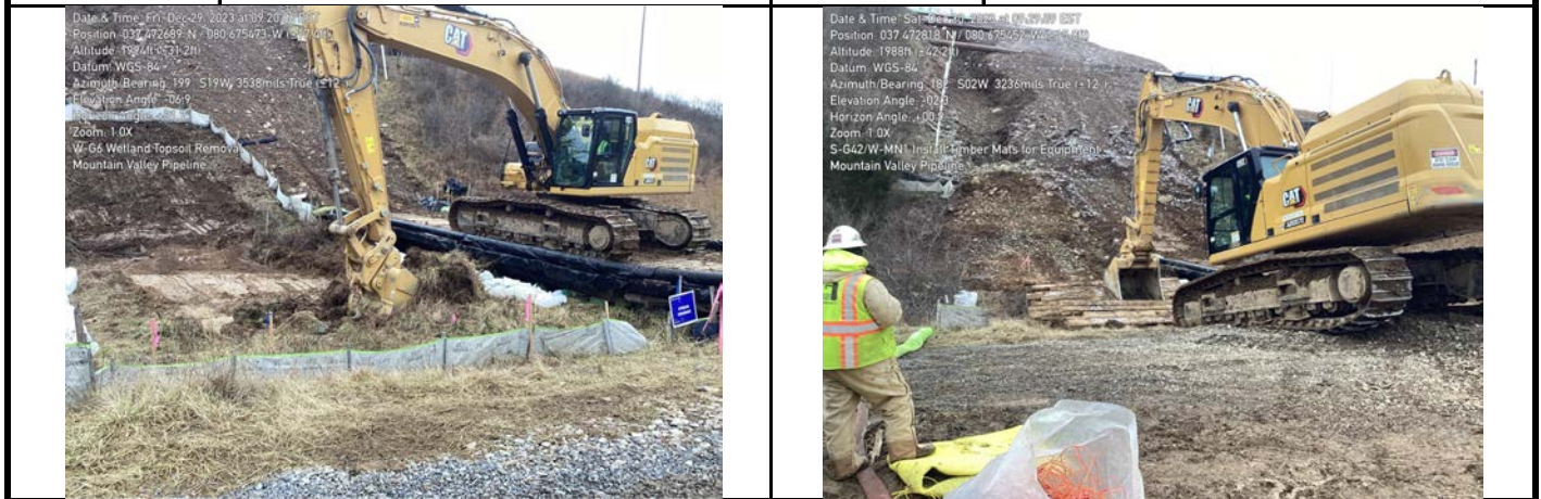
GPS Location See Photo GPS Location See Photo Description Photo 1: Excavation of top 12 inches of topsoil from aquatic resource. Description Photo 2: Installing timber mats to minimize compaction during excavation.
