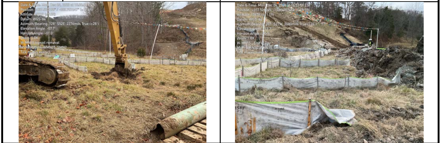
GPS Location See Photo GPS Location See Photo Description Photo 1: Excavation of top 12 inches of topsoil from aquatic resource. Description Photo 2: Aquatic resource post blast.
