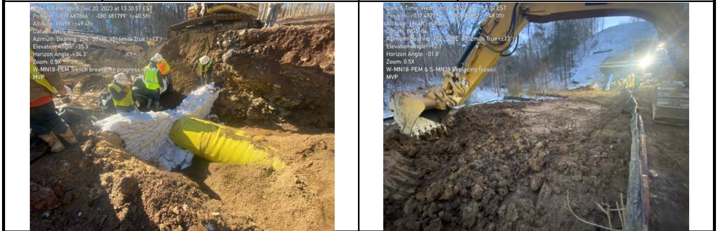
GPS Location See Photo GPS Location See Photo Description Photo 5: Constructing trench breaker. Description Photo 6: Restoring topsoil.
