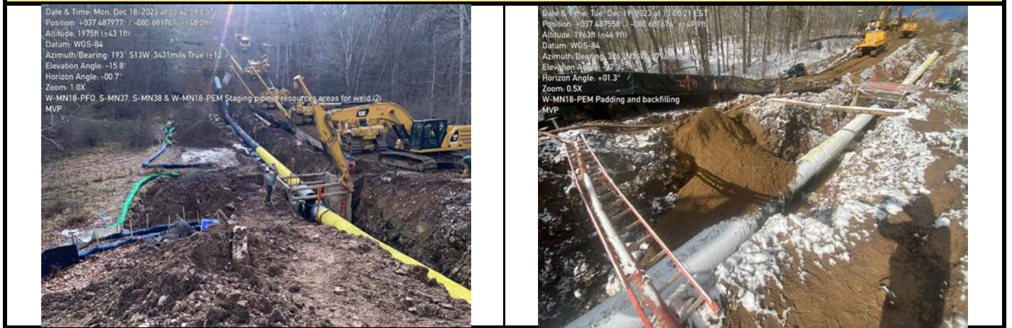
GPS Location See Photo GPS Location See Photo Description Photo 3: Staging pipe in resource area for welding. Description Photo 4: Padding and backfilling.
