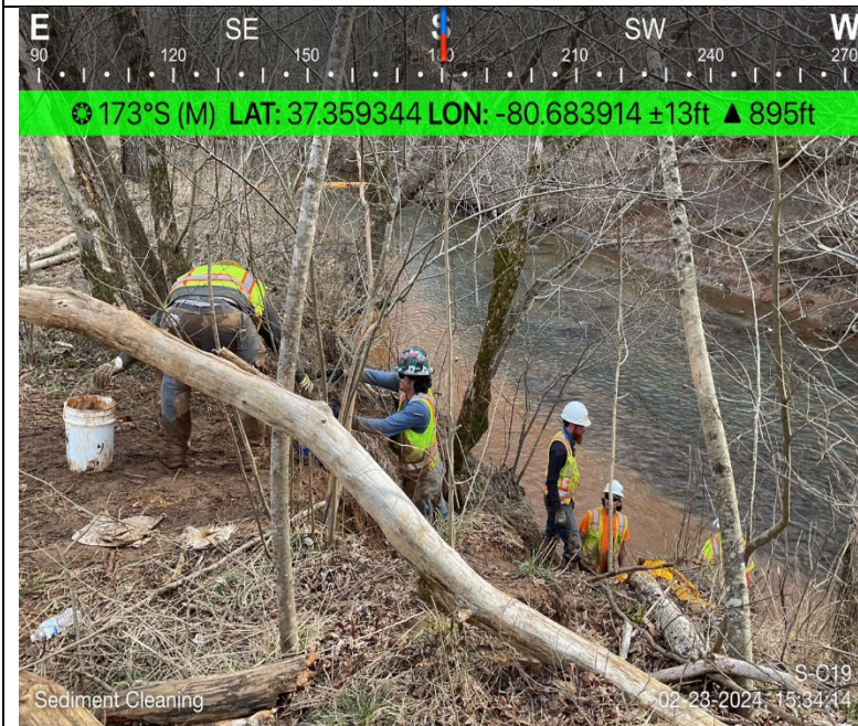
Photo Description: Cleanup of sediment from downstream area from dewatering structure runoff.
