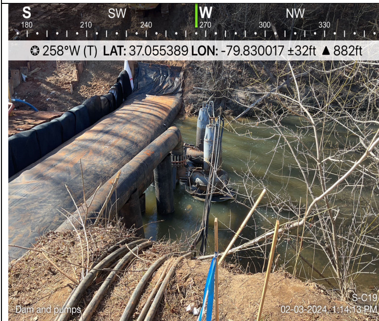
Photo Description: Bladder dam and two 24-inch pumps used for dam and pump around.
