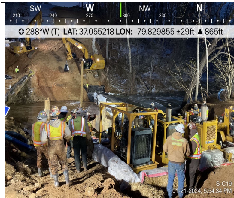
Photo Description: Tried to use back up pumps to hold water off bladder.
