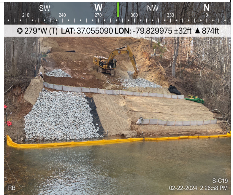
Photo Description: Installation of rip rap along stream banks to aid in long-term stability of pipeline crossing.
