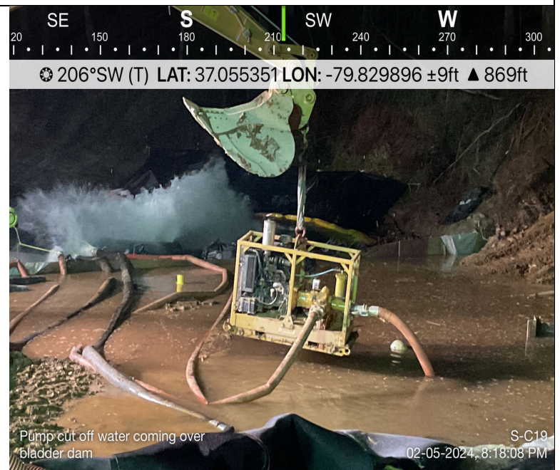
Photo Description: Holding pump in air so stream does not contact or contaminant stream. Streamflow entered into the workspace and discharge downstream.
