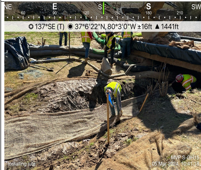
Photo Description: The stream bed and its banks were stabilized with biodegradable jute.
