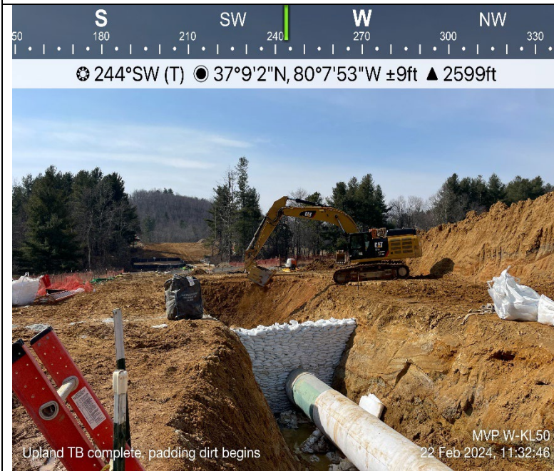
Photo Description: An upland trench breaker was installed, and the soil was padded during backfill.
