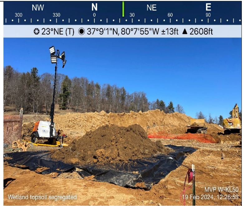
Photo Description: The wetland topsoil was segregated and stockpiled on top of Geotech fabric.
